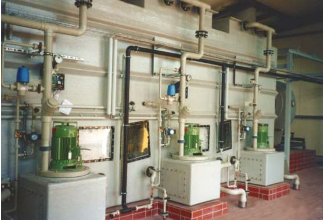
3-stage Cross flow scrubber, Material FRP
